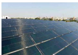
Smaller projects have also seen solar installed in court complexes and the Public Authority for Applied Education and Training's Ardiya campus.
